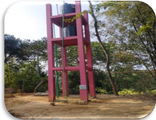
Image 3.10: Water tanks installed to ensure safe and clean drinking water supply
