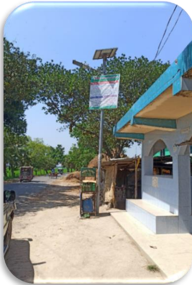
Image 3.3: Solar Street Light, Mahadevpur Upazila, Naogaon
