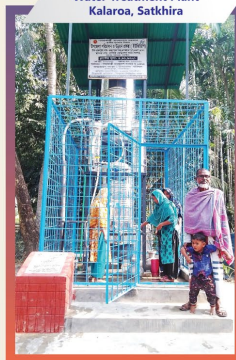
Water Treatment Plant Kalaroa, Satkhira
